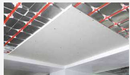
Installation and fitting of plasterboard sheets on the support structure after pressure test performed according to the rules in force
